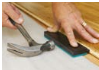
Floating a floor just means the boards are laid loose over the subfloor if they're a clic system, when floating a tongue & groove, the joints must be glued.
