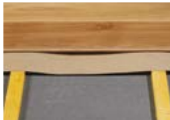
Tongue and groove planks can be secret nailed to a suitable existing timber subfloor.
